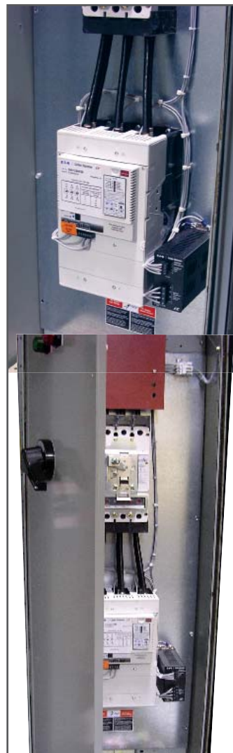
Soft-start retrofit for 250 HP
