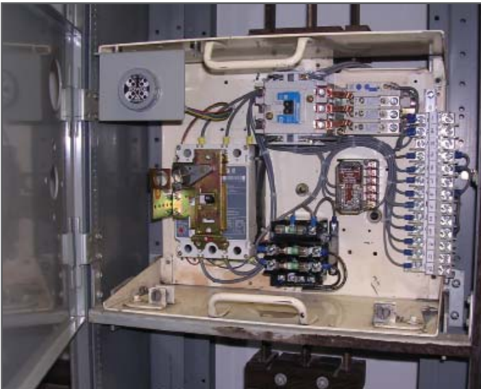
Retrofitted Cutler-Hammer 9800 with power monitor.
